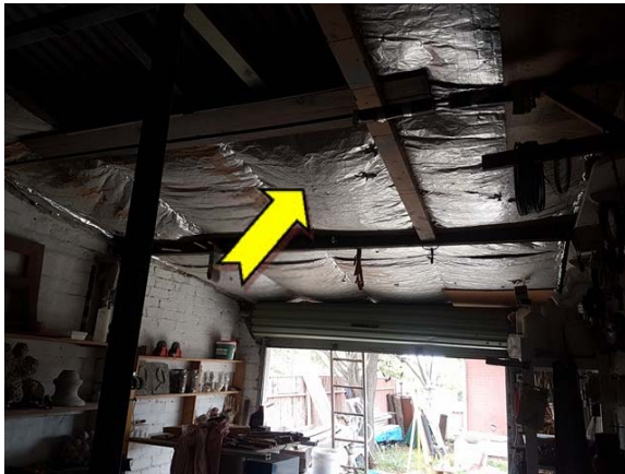
Photo 9. Interior, shed, throughout, insulation – suspected SMF sarking insulation material.
