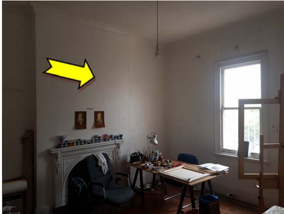
Photo 13. Interior, level one, walls – suspected lead-containing white upper paint systems.
