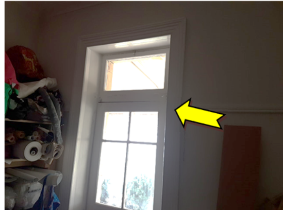
Photo 14. Interior, door and window frames, throughout – lead-containing cream upper paint systems
