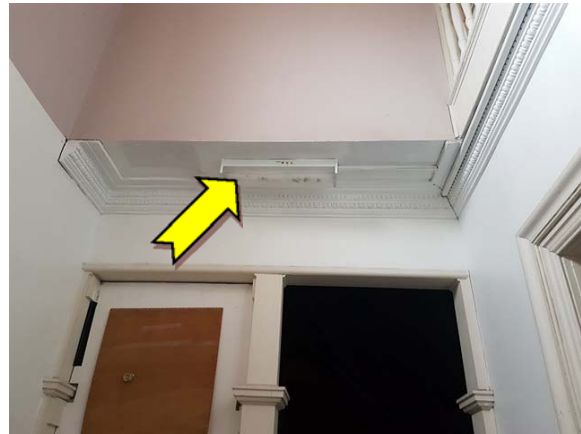
Photo 10. Interior, throughout, single tube fluorescent light fitting – suspected PCB-containing capacitor.
