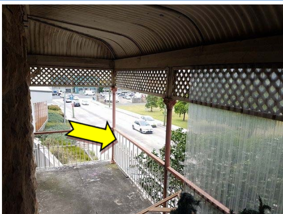
Photo 11. Exterior, level one, verandah, beams – suspected lead-containing pink and white upper coloured paint systems.
