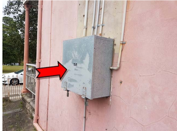
Photo 2. Exterior, ground level, south-east elevation, electrical box – suspected asbestos-containing bituminous backing board.
