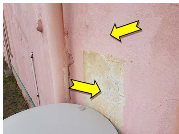
Photo 12. Exterior, walls, throughout – lead-containing cream lower paint systems and suspected lead-containing pink upper paint systems.
