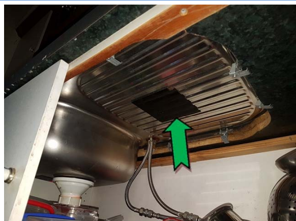
Photo 6. Interior, ground level, kitchen, under sink, sink pad – non asbestos-containing bituminous material.
