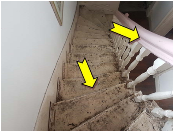
Photo 15. Interior, staircase, stairs and hand rail – lead-containing cream upper paint systems and suspected lead-containing pink upper paint systems.
